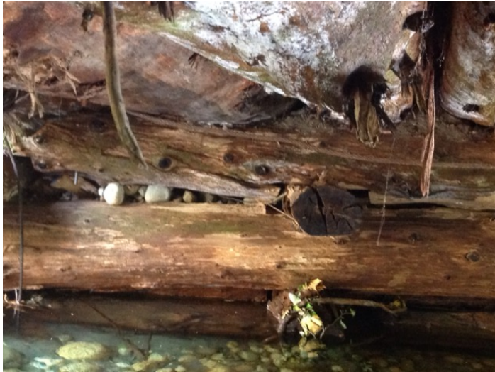
top log on left crib cracking horizontally
